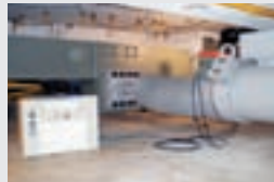
① Variable damper installed
