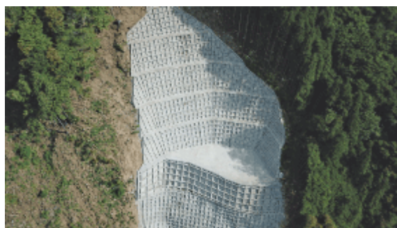
Slope Stabilization Works on the Kawatsu-Koya Prefectural Road (Yoshino District, Nara Prefecture)
